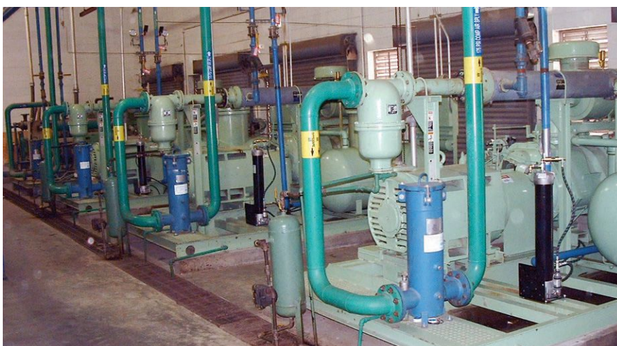
Figure 1. Air compressors are a common sight in most industrial facilities. Figure courtesy of Fluid Metrics.
